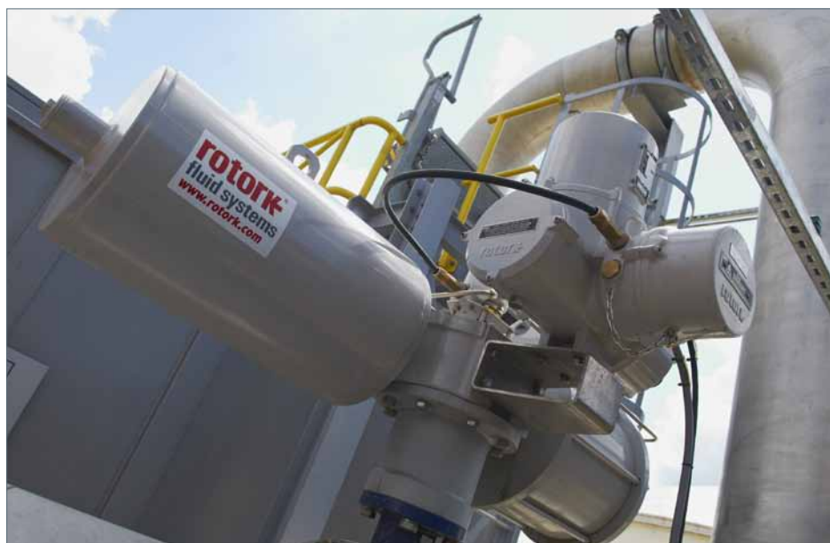
A Rotork Skilmatic EH electro-hydraulic actuator on safety related fail-safe valve duty at Vopak Phase 8.
