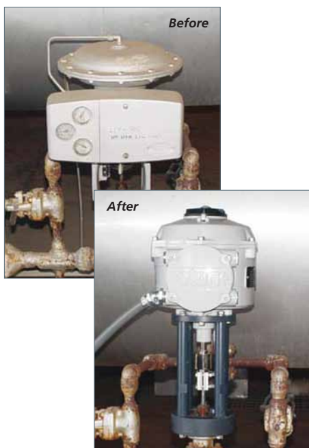
Pictured above is a before and after photo showing how a Rotork all-electric CVA actuator (bottom right) was retrofitted to replace a traditional control valve actuator (top left) in a feed water heater level-control application at a large Arizona power plant.
