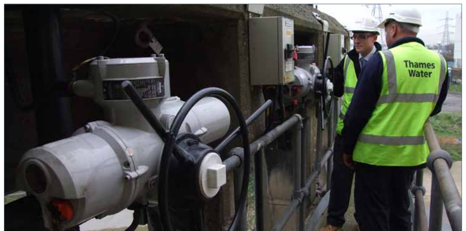
Some of the Rotork IQ Pro intelligent electric actuators on the inlet penstocks at Beckton sewage treatment works.
