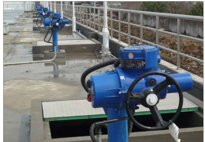
Rotork IQ Pro actuators installed on filter bed valves at Wuxi.
