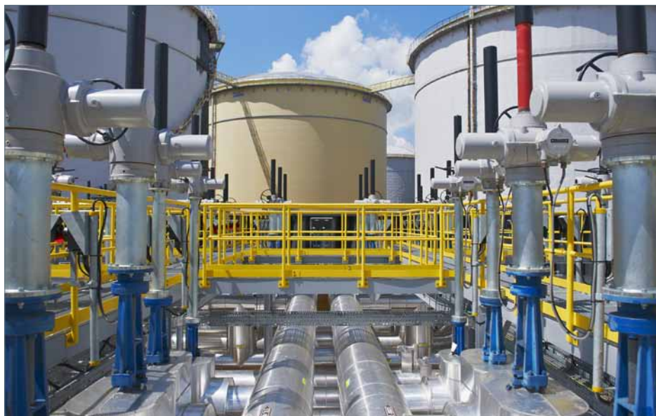
Above and below - Rotork IQ Pro valve actuator installations at Vopak Phase 8.
