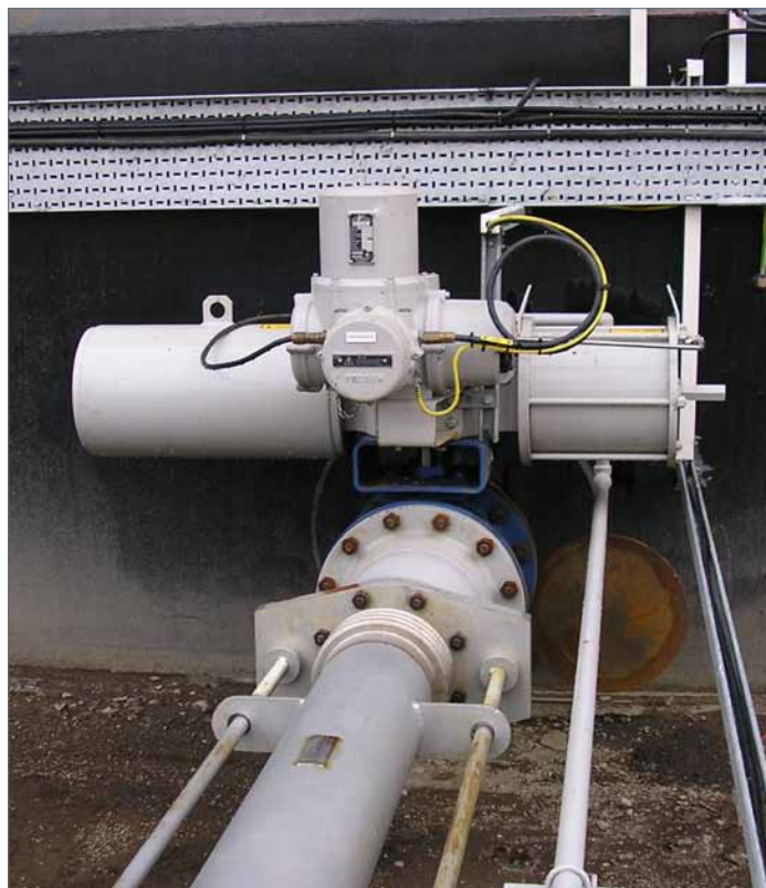
At this refinery in Scotland gate valves have been replaced by triple-offset butterfly valves with Skilmatic EH fail-safe electro-hydraulic actuators for ROSoV duty.
