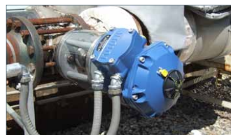
Pictured above is a Rotork quarter-turn control valve actuator (model CVQ 1200) in a NEMA 6 enclosure at New Hampshire power plant, USA.
