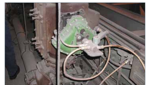
The ash hopper rotary gates at the White Bluff Generating Station before and after the retrofitting of a Type K damper drive.
