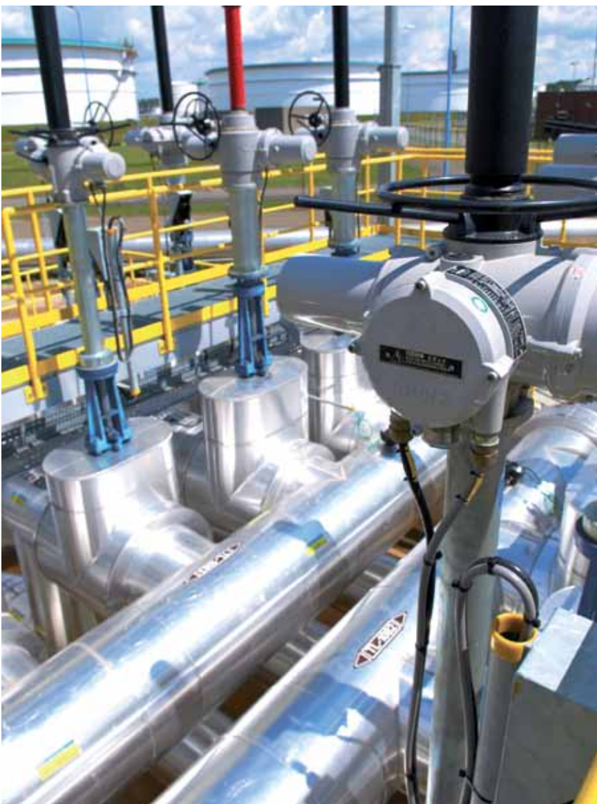
Rotork IQ actuator installations at Vopak Phase 8
