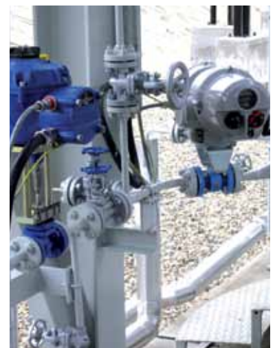
IQT and CVA actuator on new gas dehydration units in Transylvanian Romania
