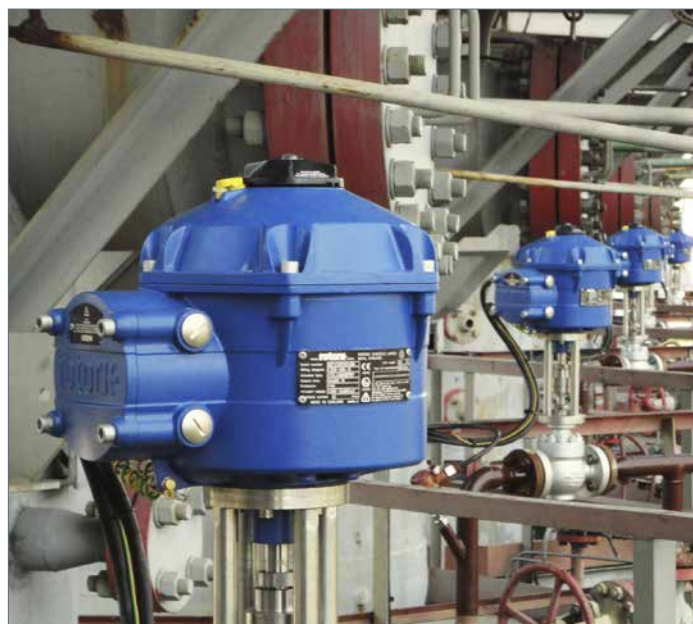
Some of the Rotork CVA actuators installed on the Bilche-Volytsa compressor station.
