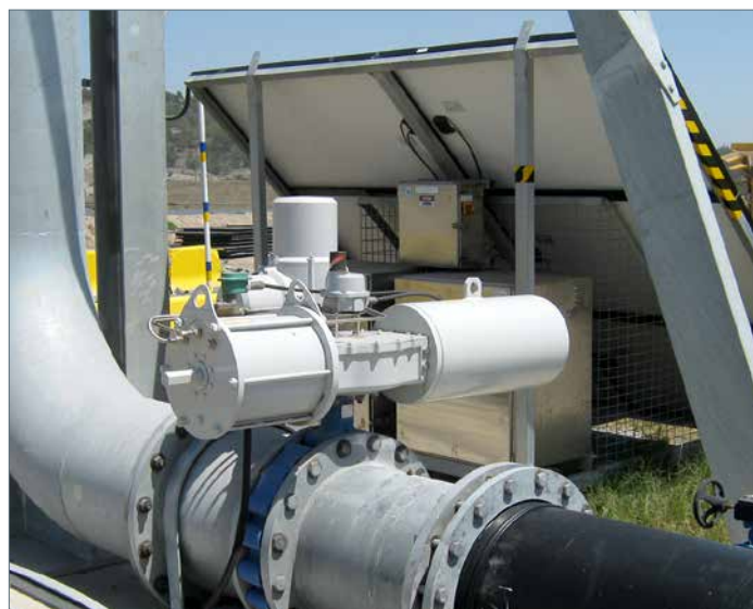
The Rotork Skilmatic Pro electro-hydraulic valve actuator installed on the Water Cart Fill Point. Solar panels seen in the background provide the renewable energy source to operate the actuator.
