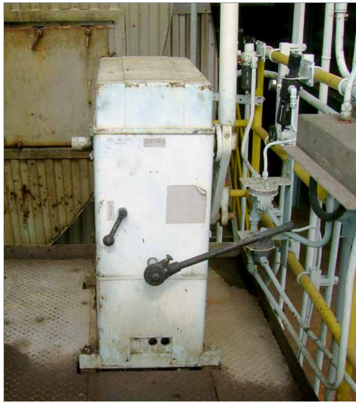
An obsolete ID fan inlet damper drive in need of replacement on Unit 1 at the Florida Power & Light Manatee Station.
