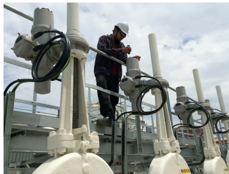
An engineer checking the commissioning settings on an IQ3 at a storage tank facility in Malaysia
