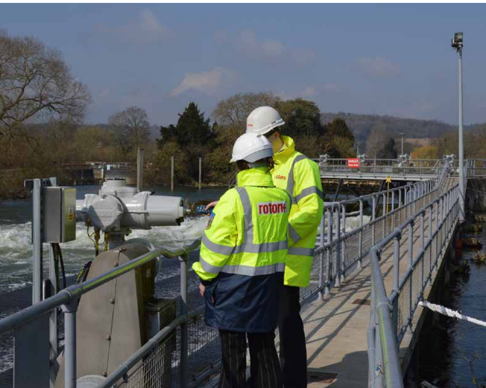
New junction boxes enable existing cabling to be used, avoiding additional expense.
