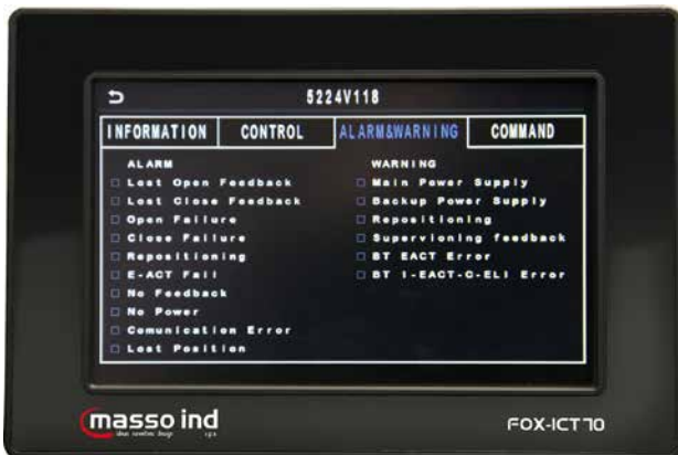
5. ALARMS & WARNINGS ACTIVE on VALVE
