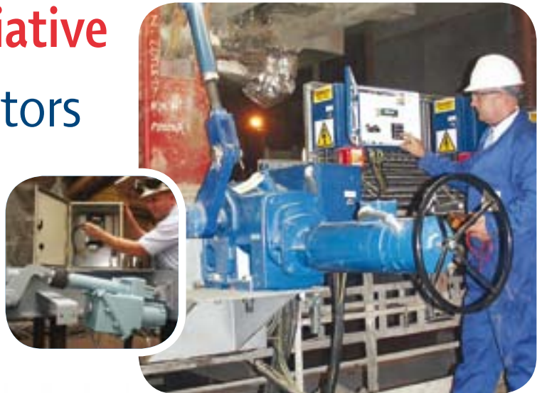
One of the SM6000 secondary air damper actuator installations at Drax.
