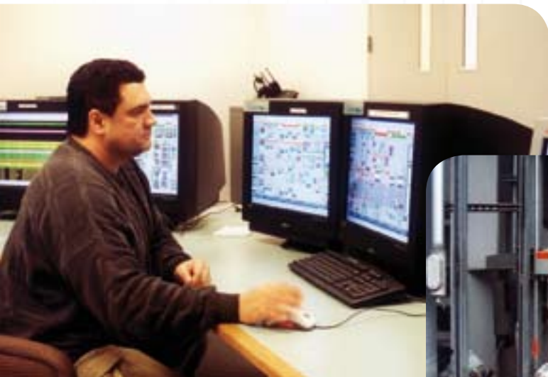
Above: When market conditions for electricity are favourable, Control Room Operator Gene Vasquez can initiate fully automated plant start-up at his computer screen. The electricity that is produced is distributed via existing transmission lines.
