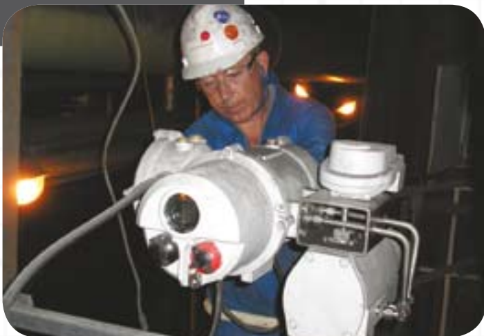
An engineer completes the commissioning of a Rotork Skilmatic actuator at Longannett.
