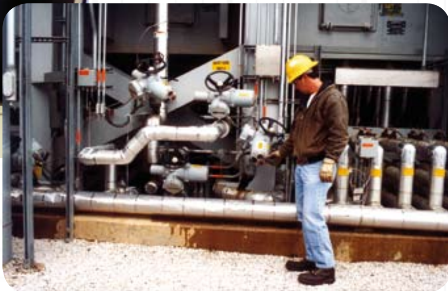
Right: Lead Maintenance Technician Bucky Ray likes the IQ infrared setting tool for troubleshooting. He can use it to easily check valve status and/or change torque and position limit settings without having to remove the IQ's covers.
