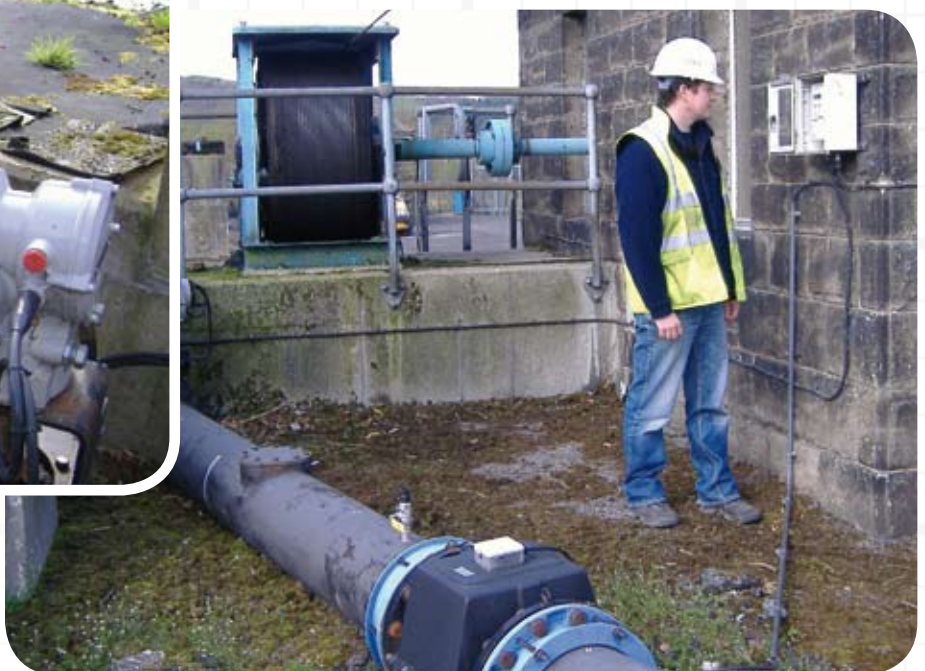
Right: Inlet installation showing the flowmeter in the foreground, the signal from which is linked to the Rotork actuator via the local control and indication panel mounted on the wall.
