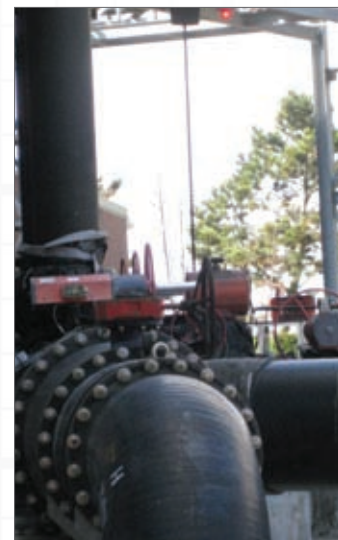
Remote Control actuators controlling the flow of the flood water
