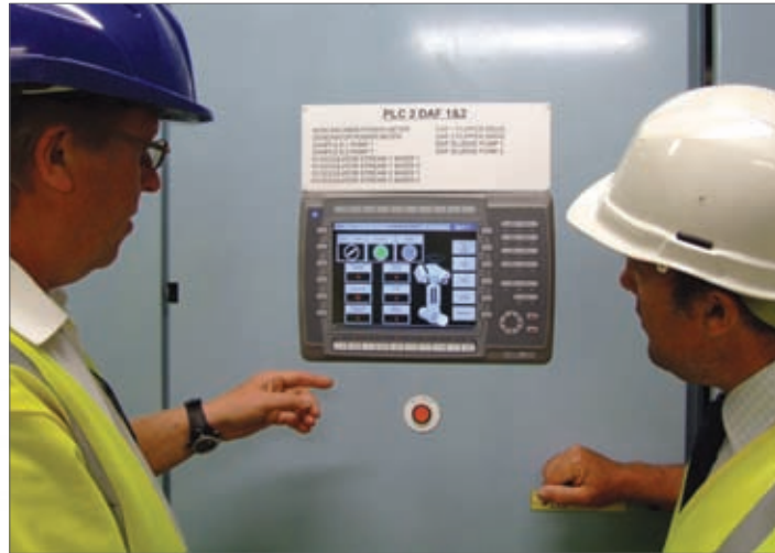
Paul Roberts from Wessex Engineering and Construction Services and Tony Scott from Rotork discuss the actuator control system and installations on the dissolved air flotation tanks in the new Maundown building
