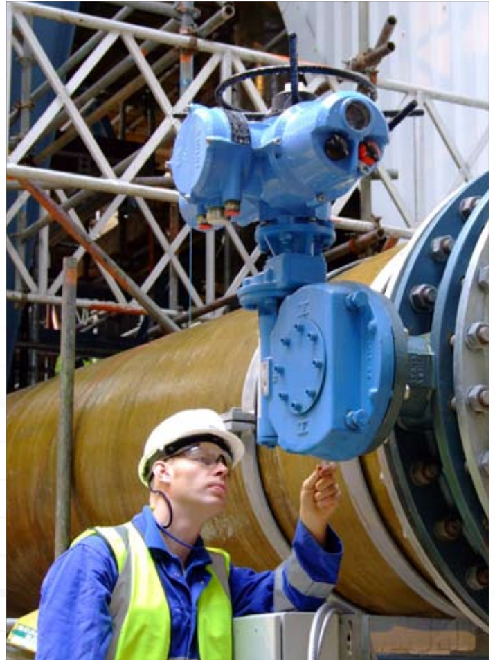
Exeeco engineer Jonathan Darker inspects IQ installations on the Ferrybridge FGD plant
