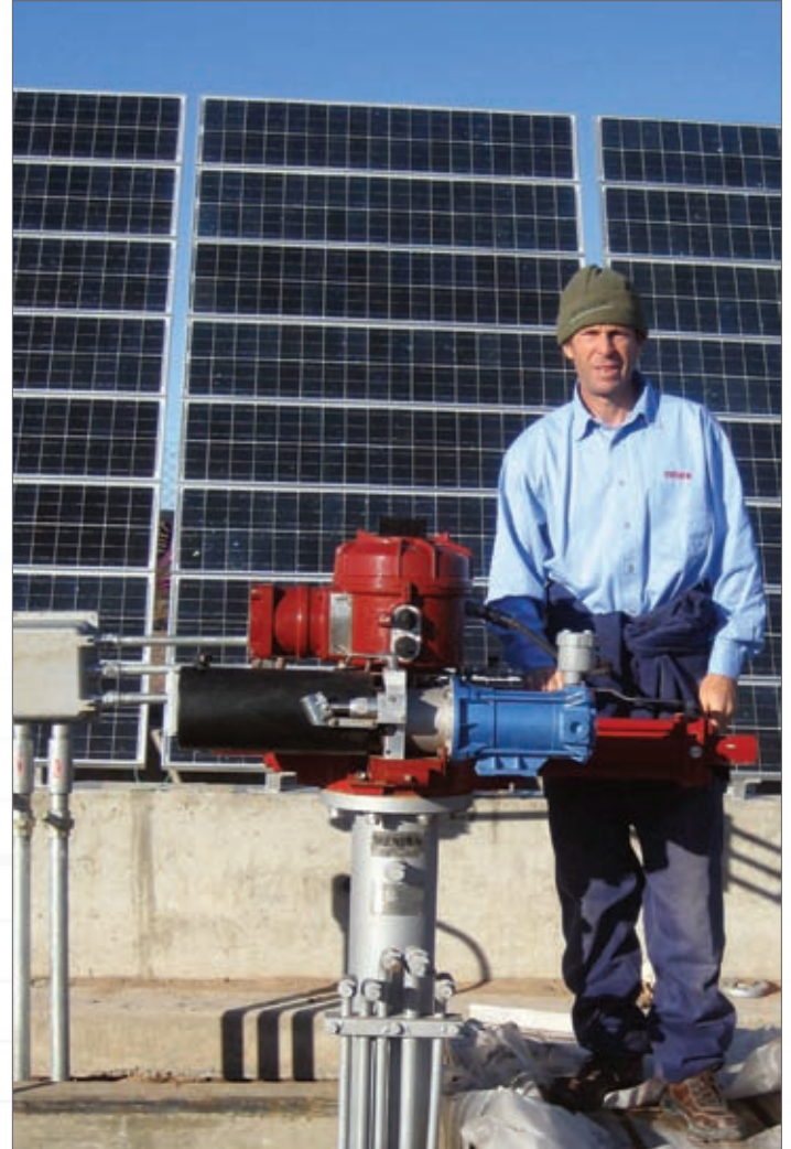
Paplo Patane from Industrias Metalart S.A. is pictured with one of the Skilmatic EH actuator installations, framed by solar panels
