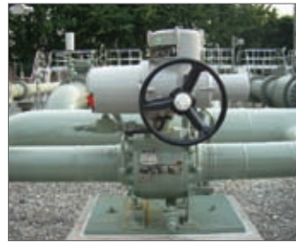
Actuators installed at one of the pipeline pump stations
