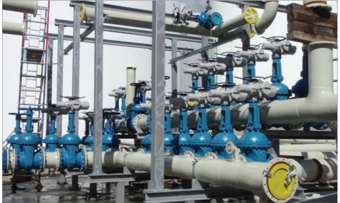
IQPro actuators installed during construction of the new main manifold at Skarvik 1
