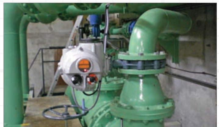
IQT actuator installed on a 150mm butterfly valve in the airport's cooling plant
