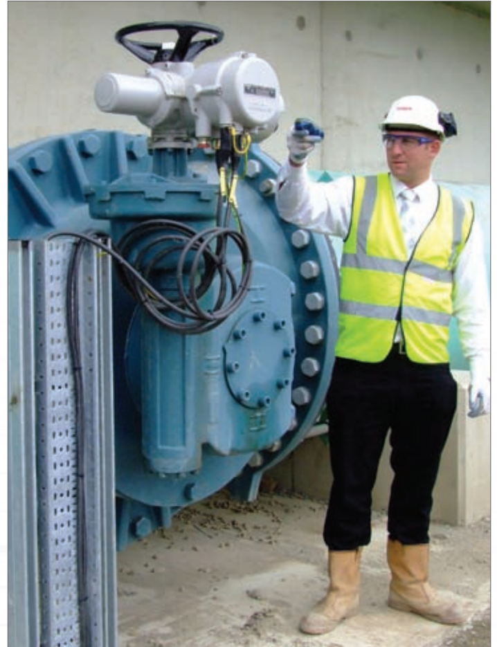
A Rotork engineer downloads valve operating data from one of the Rotork IQ Pro modulating actuators on the selector plant using the 'non-intrusive' hand tool that enables data to be transferred for analysis on a PC running Rotork IQ-Insight software. The Rotork IQM12 modulating actuators on the plant are fitted to Rotork Gears MOW9R spur/worm secondary gearboxes.
