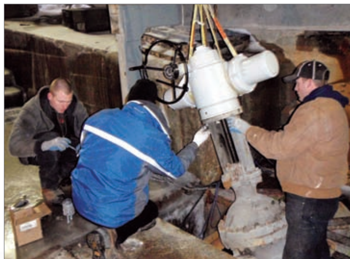
Retrofit work in progress on one of the valves, deep in the bowels of the structure.
