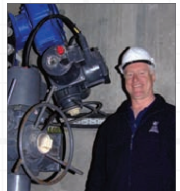
Senior Maintenance Engineer Richard Parker with two of the Rotork IQ actuators on the pipework branch leading to the two sea locks.
