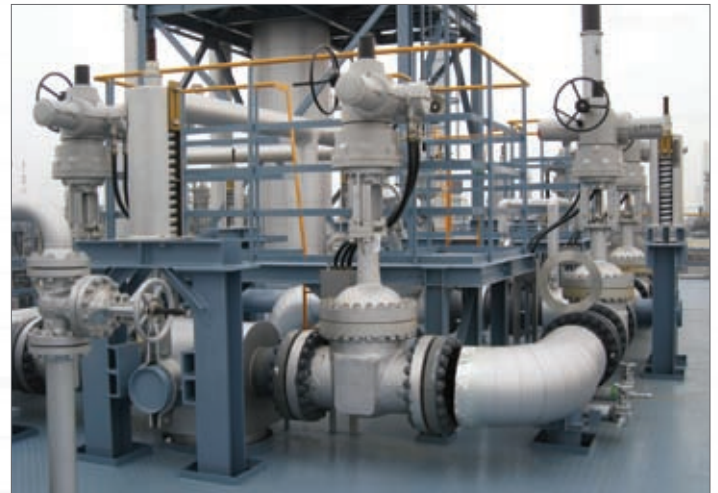
Rotork IQPro valve actuators with thrust compensators installed on the new Mitsui Chemicals plant.
