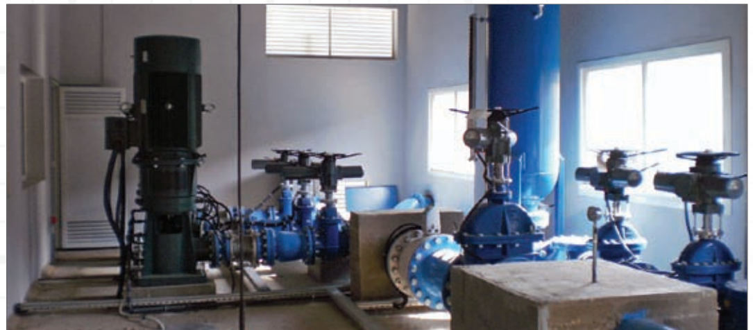
Rotork AWT actuators installed at the Qattine Azar clean water distribution network.
