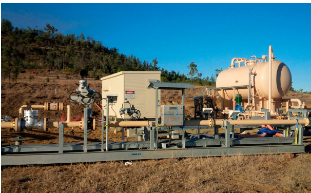
Figure 2. Rotork actuator installation at a wellhead and separator skid in Australia.
