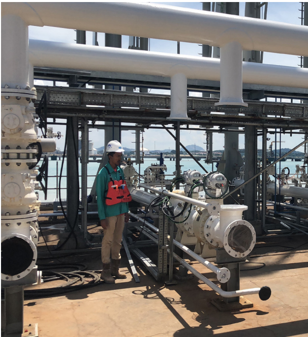
Figure 3. IQ3 actuators at the Pengerang terminal, Malaysia, during the installation stage.
