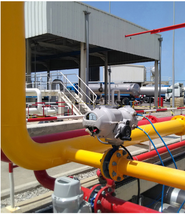
Figure 1. Rotork IQ3 intelligent electric valve actuators with Pakscan digital control network at Horizon Tangiers Terminals S.A.
