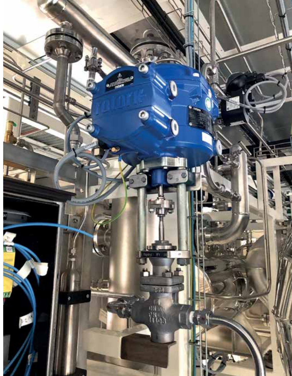
A Rotork CVL actuator on an electrolysis skid
