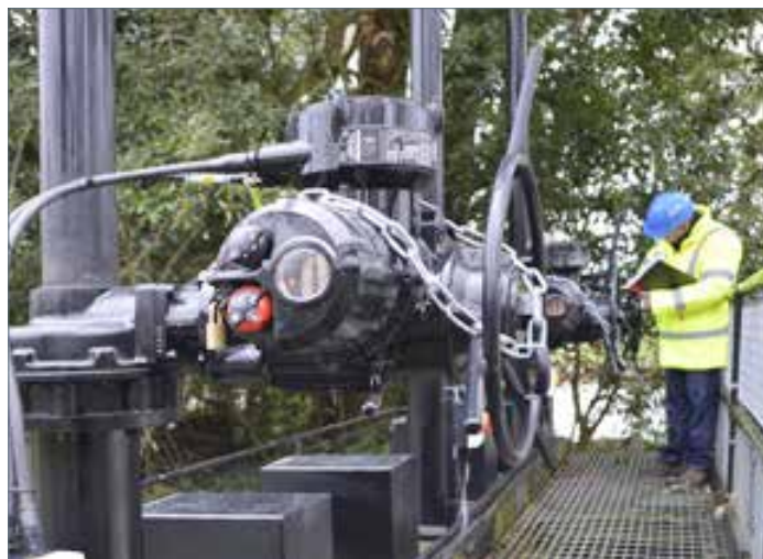
Final inspection in progress following completion of the automation upgrade of Canford Sluice.
