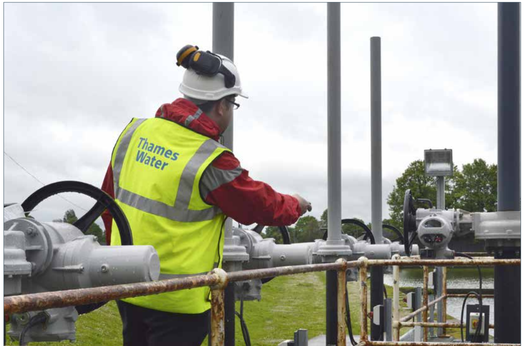
David West, Thames Water's West London Abstraction Engineer, uses the hand held setting tool to operate an IQ3 actuator at the upgraded reservoir inlet site.
