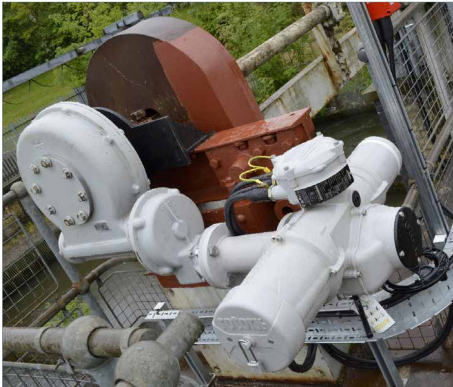
One of the Rotork IQ3M actuator and gearbox installations on the river gates; the actuator is fitted with a vandalproof cover to prevent unauthorised local operation.
