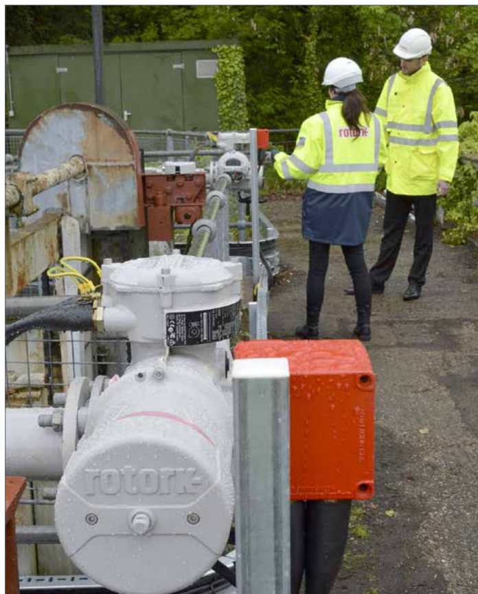
Using the non-intrusive setting tool, Rotork Site Services engineers confirm the commissioning settings on an IQ3M actuator.
