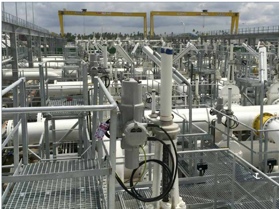
A 'sea' of Rotork actuated valves in one area of the Pengerang Terminal.
