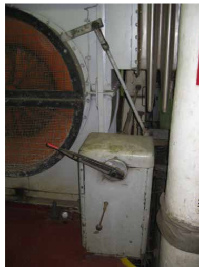
Existing, inefficient pneumatic damper controllers.
