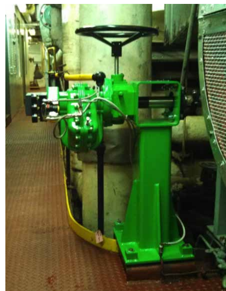
Installed Type K damper drive unit.
