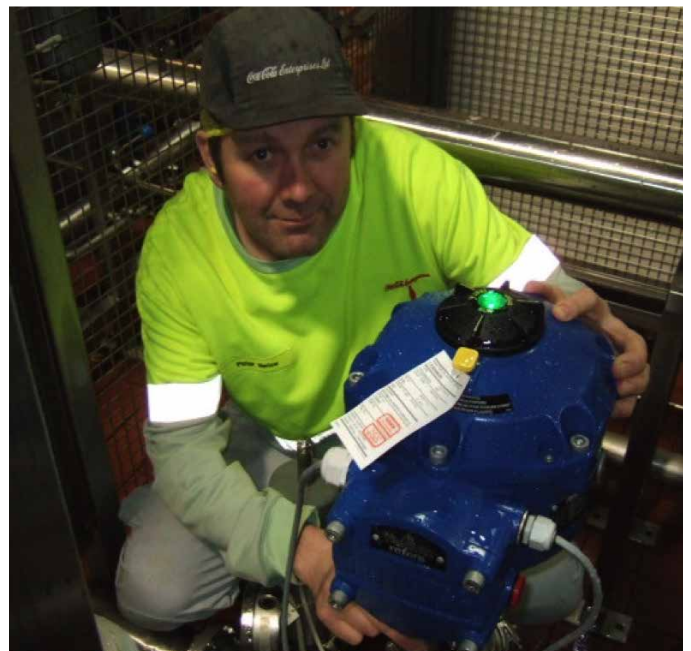
CVA actuator installed at Coca-Cola Enterprises.
