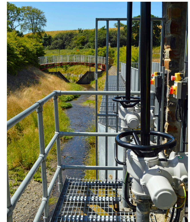
Above: The River Mwidan flood alleviation scheme, showing two of the new Rotork actuators in the foreground and the V notch weir in the background. The over-spill grid is in between.
