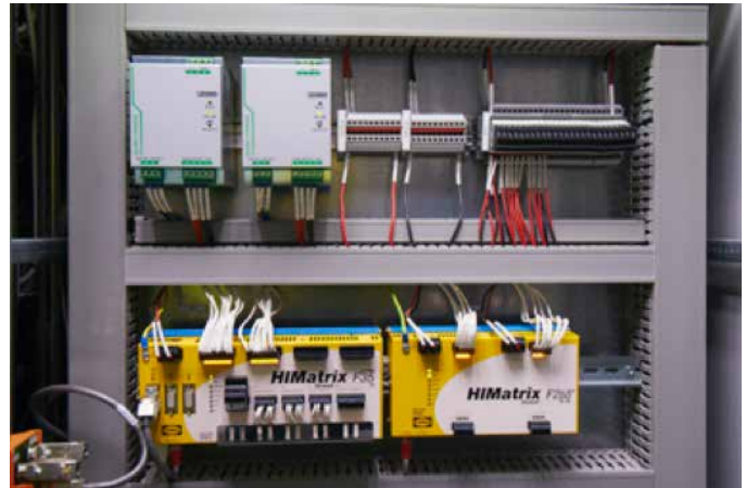
ESD separately hardwired PLC control station at BTT.
