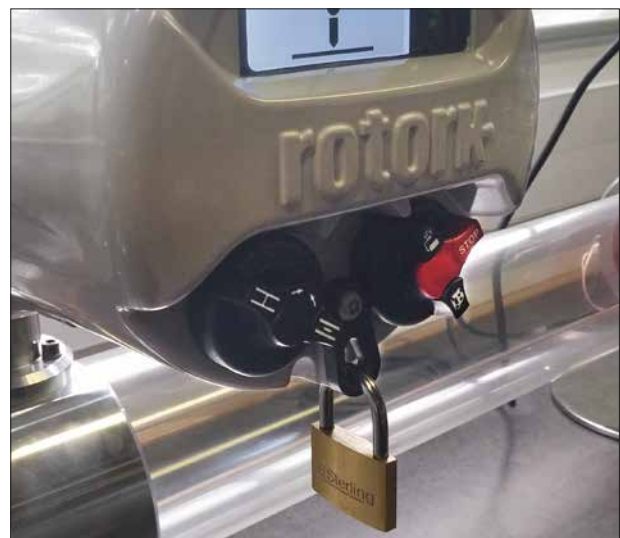
Fig 7.2. IQ3 control selector padlocked in "Remote"
