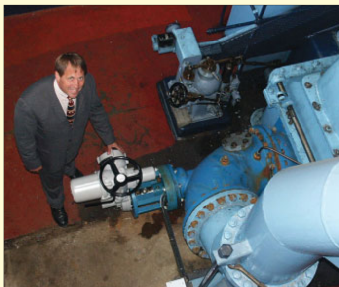
Rotork IQM actuator operating the linear water inlet valve on one of the turbines at Mary Tavy. Far right: Rotork d.c. actuators on the main turbine inlet valves.
