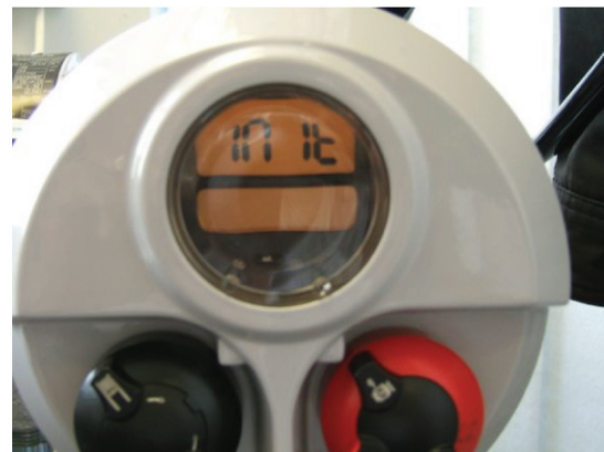
Commissioning mode initialised
