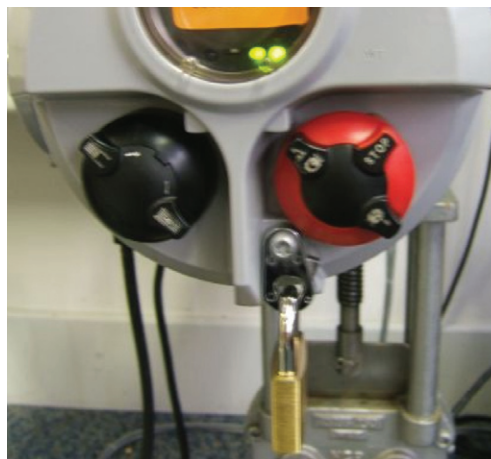
Fig 3 IQ/IQT control selector padlocked in "Remote"
