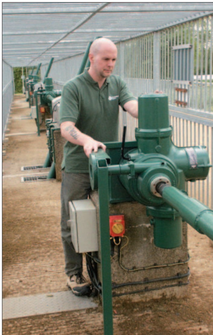
Russell Gillet, Operations Officer for the Environment Agency, inspects one of the new Rotork IQ40 actuator installations on Bedford Sluice.
