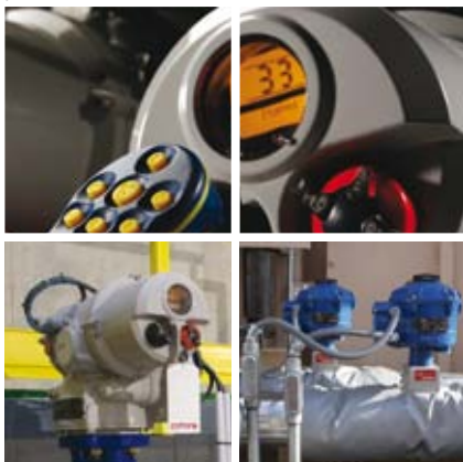
Bottom Right: CVL actuators in oil recovery plant, USA.
