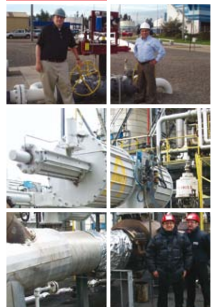
Bottom: GP actuator upgrade to improve partial stroke testing capability, Rafferia Miazzo, Sicily.
