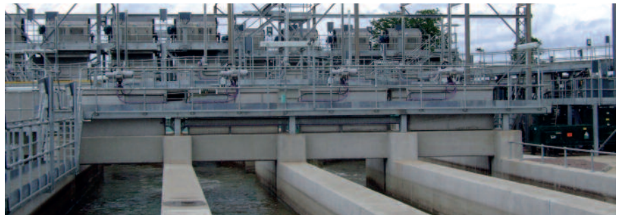
Valves are the vital components in any plant that relies on well managed flow control
