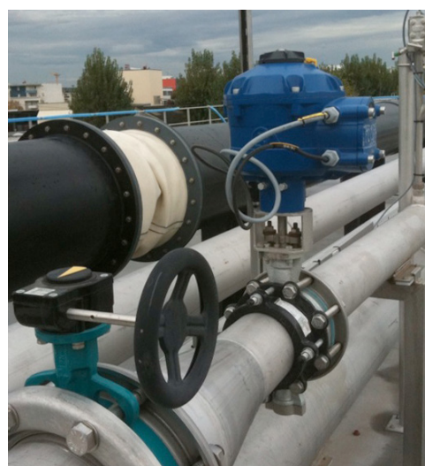
Fig 4 - A Rotork CVA actuator installed on an air supply line feeding a biogas production process.
