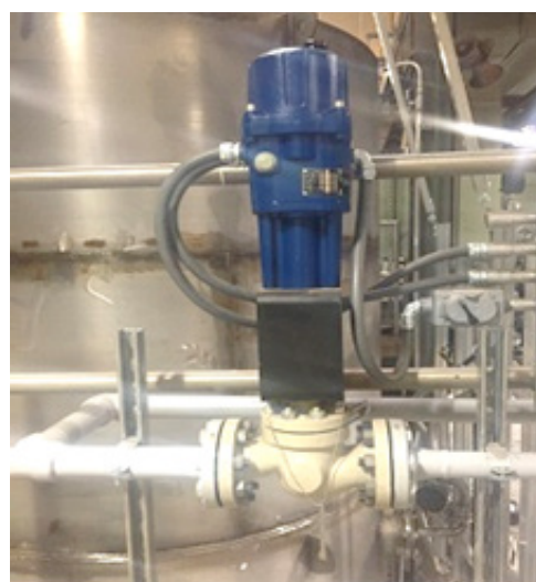
Fig 3 - Modulating electric actuator on incinerator plant in a wastewater treatment plant.
