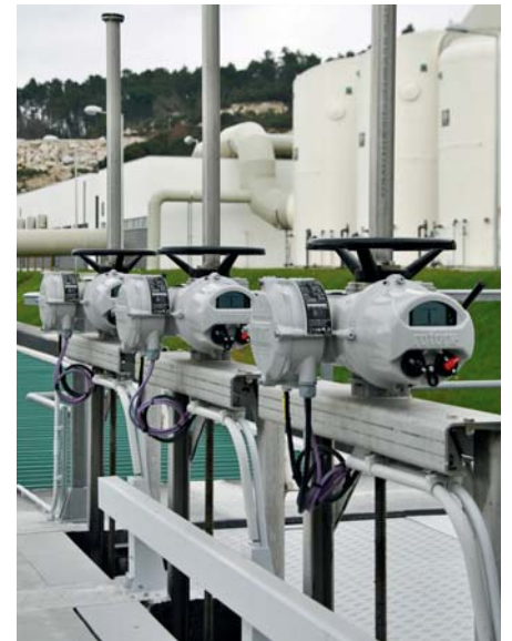
Figure 4. The Viseu Sul WWTW in Portugal is the first in the country to adopt advanced membrane filtration (MBR) wastewater treatment technology. MBR treatment plants work without the addition of chemicals and with relatively low energy consumption. Centralised process control and automation is facilitated using Profibus DP enabled Rotork IQ3 actuators to operate penstocks and butterfly valves for flow control throughout the wastewater treatment process. Extensive actuator diagnostics and configuration information is included in the data supported by the Profibus card, enabling valve profiling and diagnostic data collected by the IQ actuators to support asset management at Portugal's environmental benchmark for wastewater treatment.
