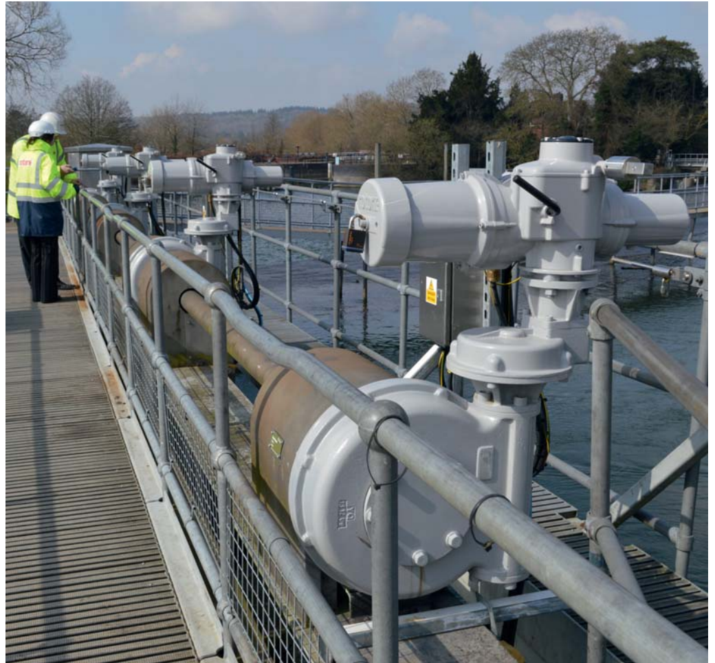
Figure 1. Rotork IQ3 actuators were chosen to provide reliable operation of radial gates that play a vital river management role on the River Thames. Reliability problems with previously installed actuators mostly resulted from inadequate environmental sealing. It was therefore decided that replacing them with double-sealed Rotork IQ3 watertight actuators would be the best solution.
