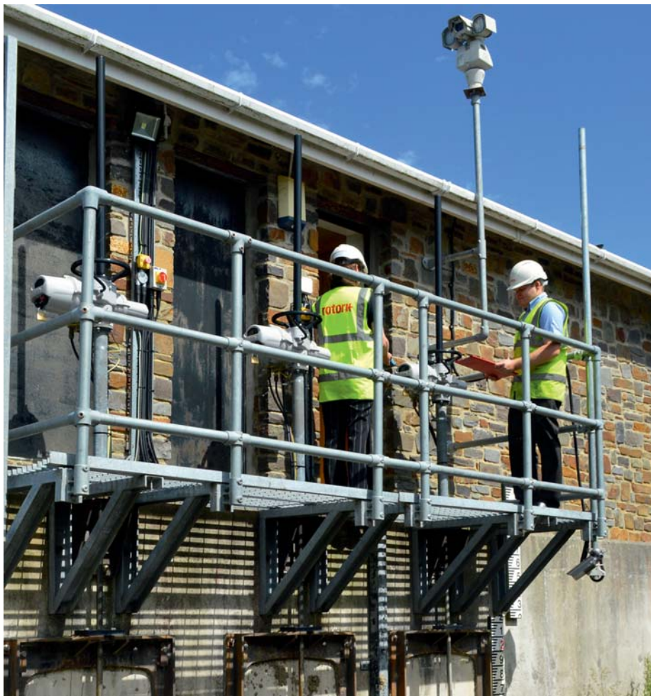
Figure 2. Rotork IQ intelligent valve actuators provide full automation of a flood alleviation scheme protecting the historic town of Cardigan in West Wales. Rotork's responsibilities included an initial survey, removal of old actuators and replacement with new, installation of a PLC control cabinet with HMI for local control and indication, interfacing with the level sensor and telemetry system and commissioning of the completed installation. Operation of the site is now fully automated and remotely monitored.
