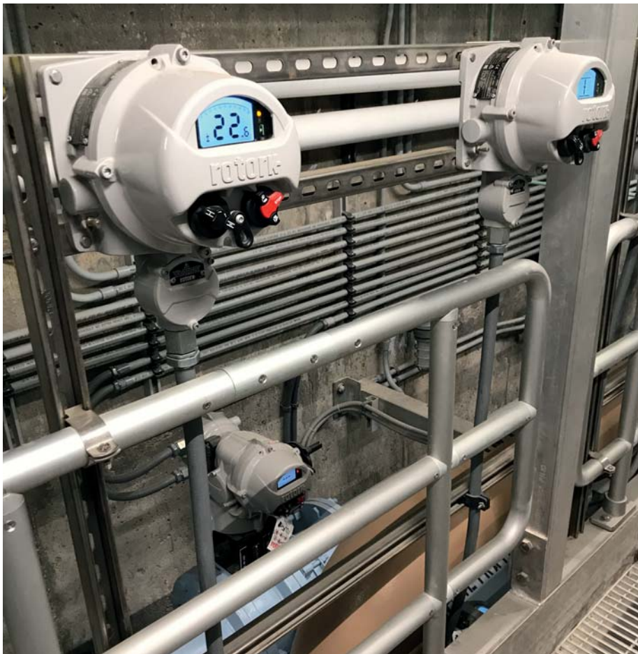
Figure 3. The valve upgrade with IQ3 actuators at a water treatment plant in Olathe, Kansas, USA, included filter plant butterfly valves in an area beneath a walkway which made it difficult to access and operate the actuators. With the Rotork actuators, the installation of Remote Hand Stations (RHS) eliminated this problem.
